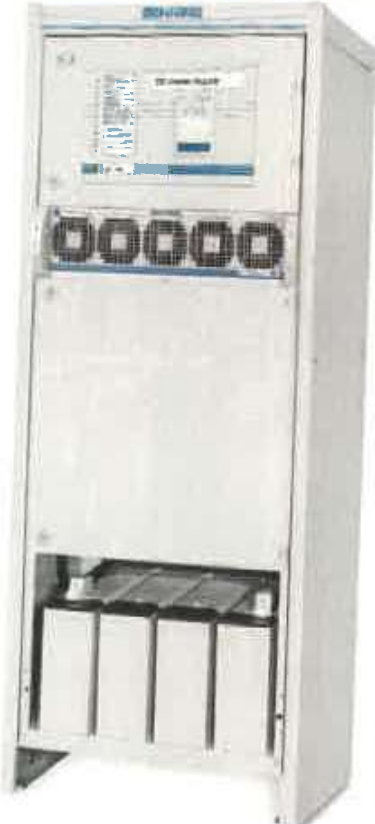
Examples of modular DC-power systems: Fig. 11: output voltage 24 V, output current 210 A
