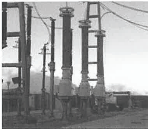
4. 420 kV Inductive voltage transformers. R.E.E. (Portugal)
